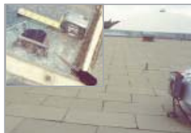
Andrew H. S. – Andrews, TX Skylight with 6” hail damage
